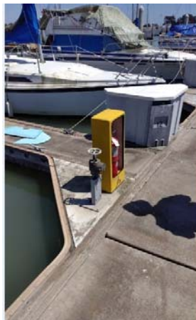
Photo 16 - Typical Fire Extinguisher and Hydrant
